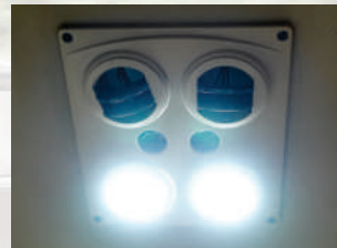
Individual AC Louvers & LED Reading Lamps
